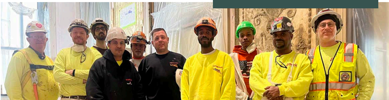
DC 9 painters and decorators restoring the historic Waldorf Astoria Hotel in Manhattan. In addition to painting, decorating, and specialty finishes, DC 9 paperhangers, drywall finishers, and glaziers helped with the restoration.
